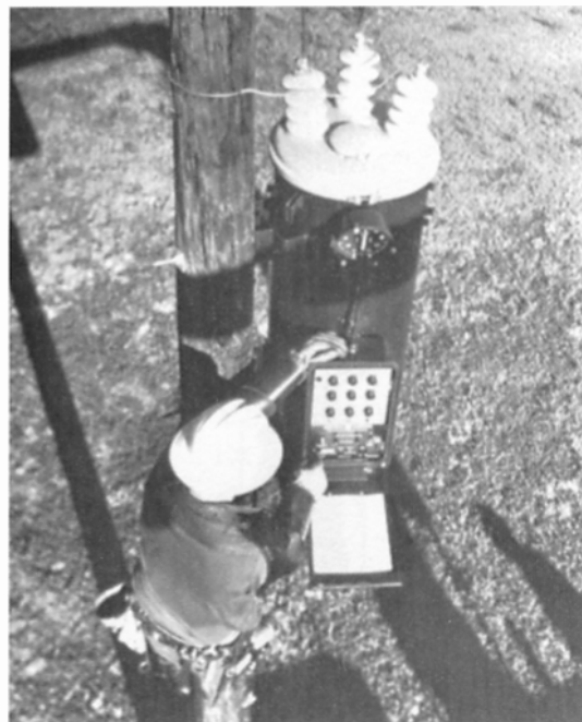
Figure 26.29 Automatic tap-changing autotransformer maintains steady voltages on long rural lines. (Courtesy of General Electric)
